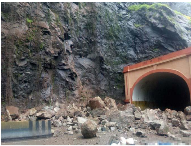
(c) Rock fall at Adoshi Tunnel
