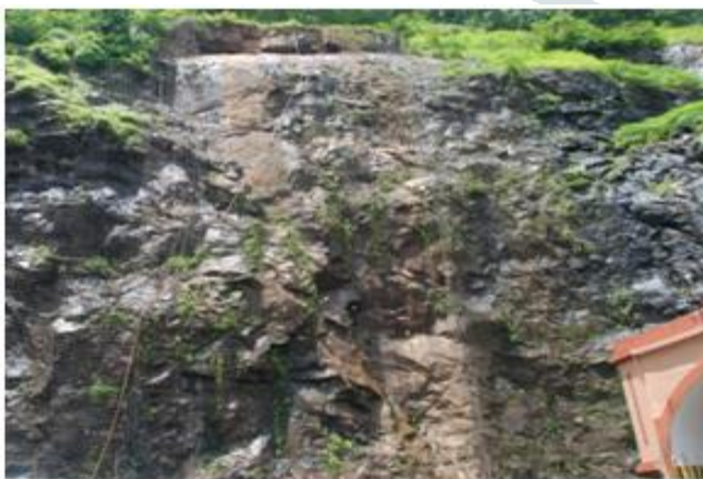
(a) View of Adoshi Hill after the distress
