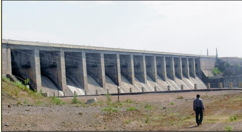
View of Sluice gates of Siddheshwar Reservoir, Roopur Camp Tq. Aundha (N), Dist. Hingoli
