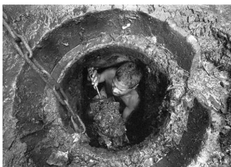
Fig. no. 1 A sanitation worker without any safety equipment. [1]
