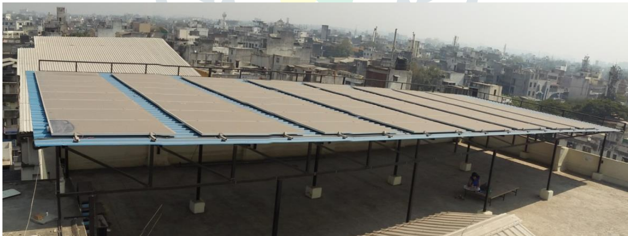
Figure 1: 20kW rooftop on grid photovoltaic solar system installed at Haribhai V. Desai College, Pune.
