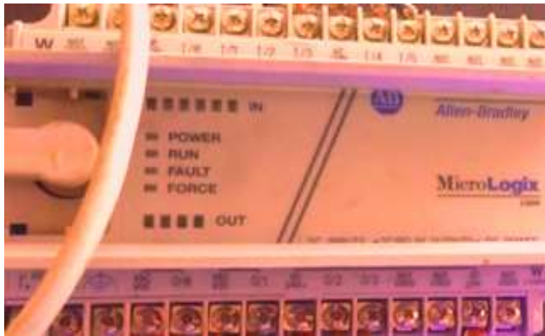
Fig 3 Hardware of PLC
