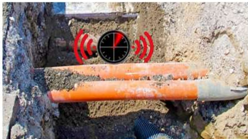
Figure 1: Picture Depicting The Fault In Underground Cables.
