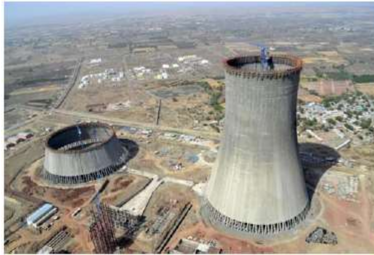
Fig. 1: Illustrates the constriction of Kalisindh thermal energy plant in Rajasthan, India containing cooling tower [5] .
