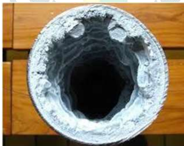
Figure 3: Illustrates the deposition of fouling material over cross section of the tubular heat exchanger[6].
