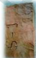
Fig.7: Photograph Showing a Customized Brick with ‘Slight’ Efflorescence on Red Marked Areas.
