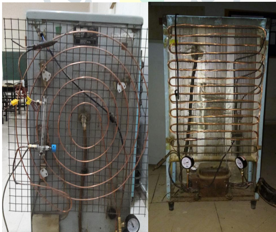
Fig. 3 VCR installed with Spiral condenser and Microchannel condenser
