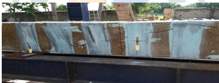
Fig.5. Failure mode of side strip beam-1
