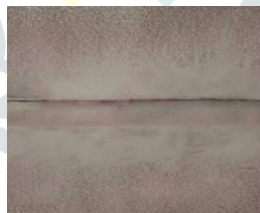
Fig 7.6: welded plate indicating less defects
