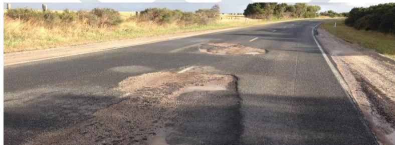
Fig. Village side damaged road
