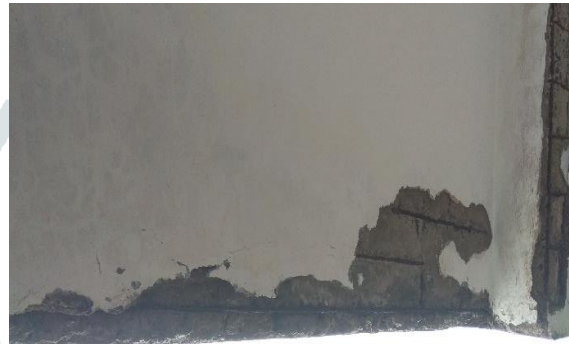
Fig 3.2 Reinforcement Expose in Cantilever Slab
