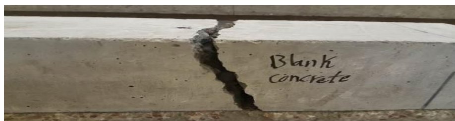
A) Fig 10. Typical fracture of unreinforced concrete
