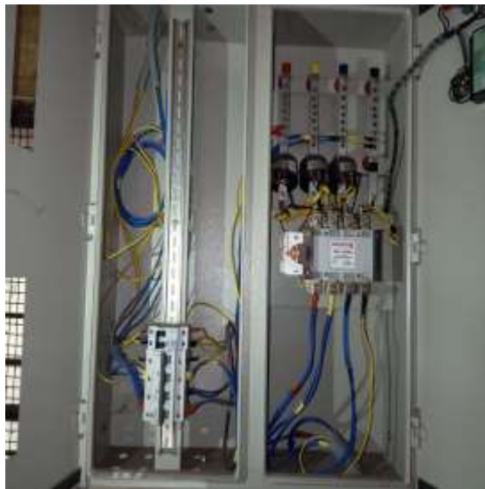
Figure5: Three Phase Distribution Board components
