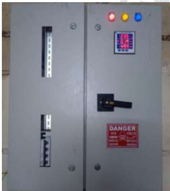
Figure6: Three Phase Distribution Board
