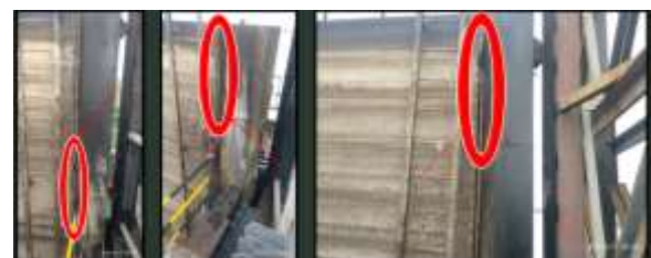
IMG 1.2 Damaged Rubber Seal
