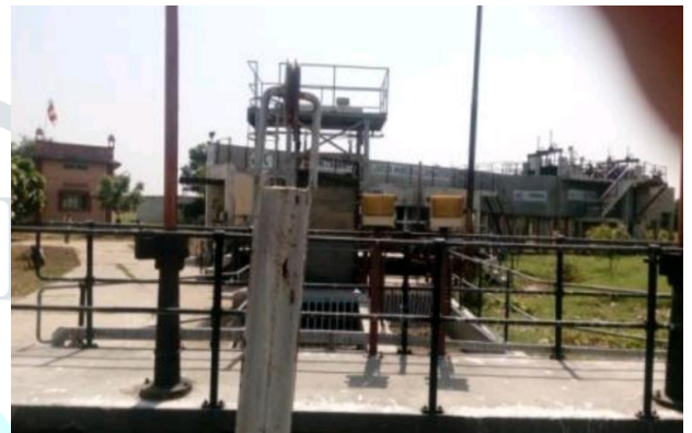
[Fig.07 Inlet Section of STP]
