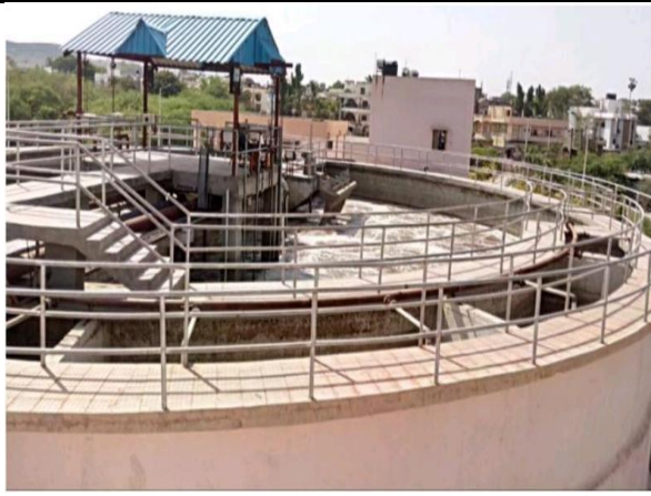
[Fig.08 Reactor at STP of Salim Ali Lake,Aurangabad]
