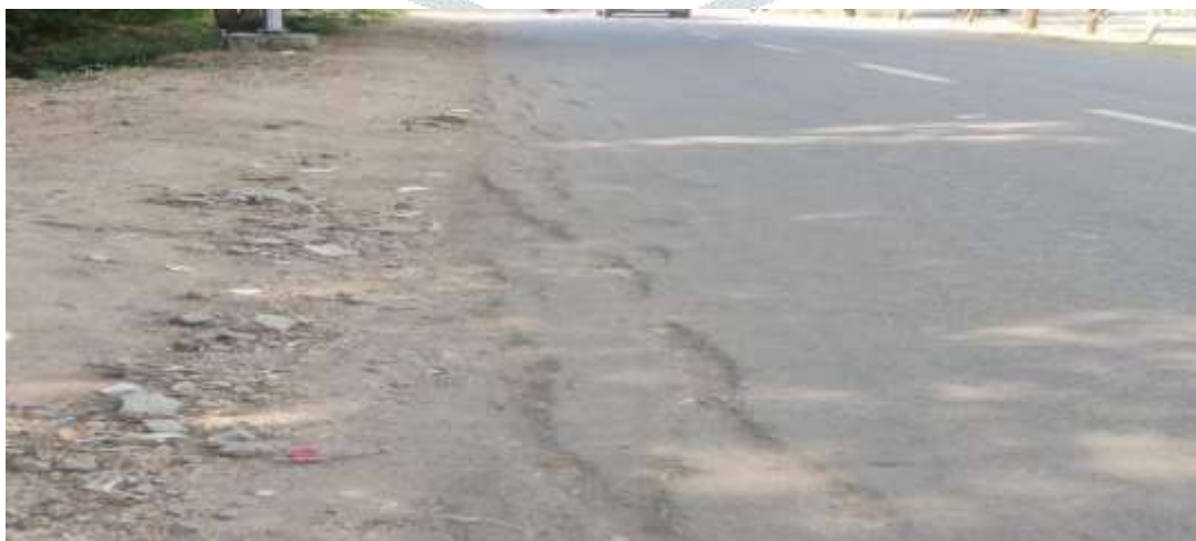
Fig: Linear cracking (longitudinal)
