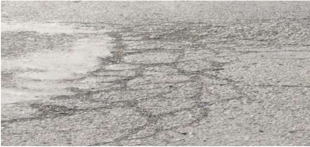
Fig: Block cracking
