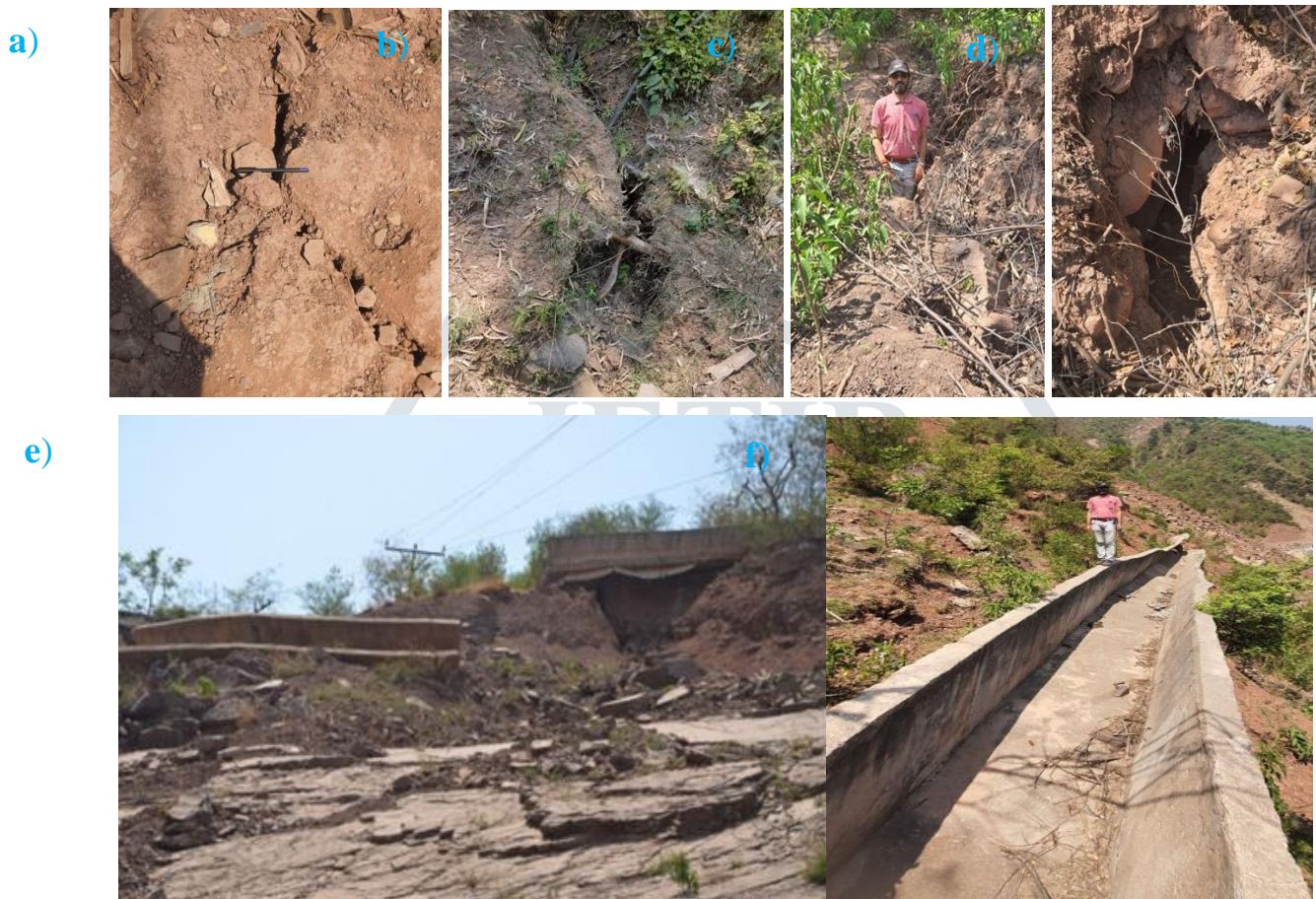
Fig. 1.2: Field photographs (a-d) showing wide open and deep cracks at the different portion of the slide; e) displaced drainage channels and f) incomplete drainage left in the sliding area.
