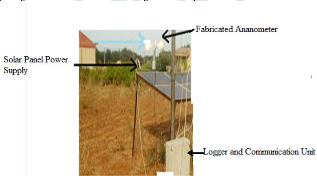
Plate 4: Deployed wind logger
