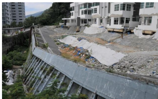
Figure 1: Collapsed Retaining wall Beverly Hills Tanjung Bungah, Penang
