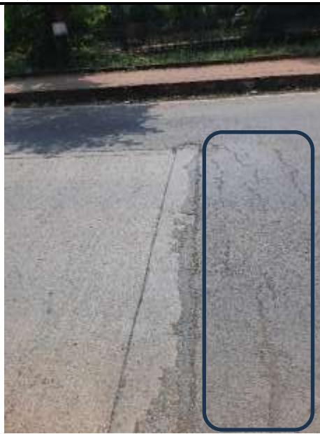
Fig. 8 Transverse cracks at the junction of R.C.C beam and Asphalt stretch.
