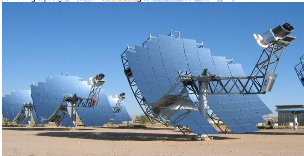
Fig. 7: Dish Sterling being used for Solar Power Production.
