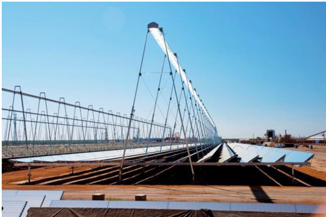
Fig. 6: Solar Park with Linear Fresnel Reflectors.
