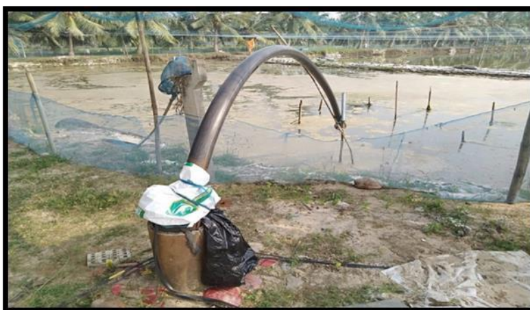
Plate 2: Bore water pump
