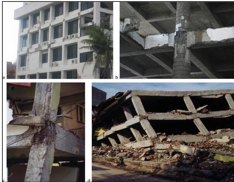
Figure 1 Structural Damages Caused by Earthquake
