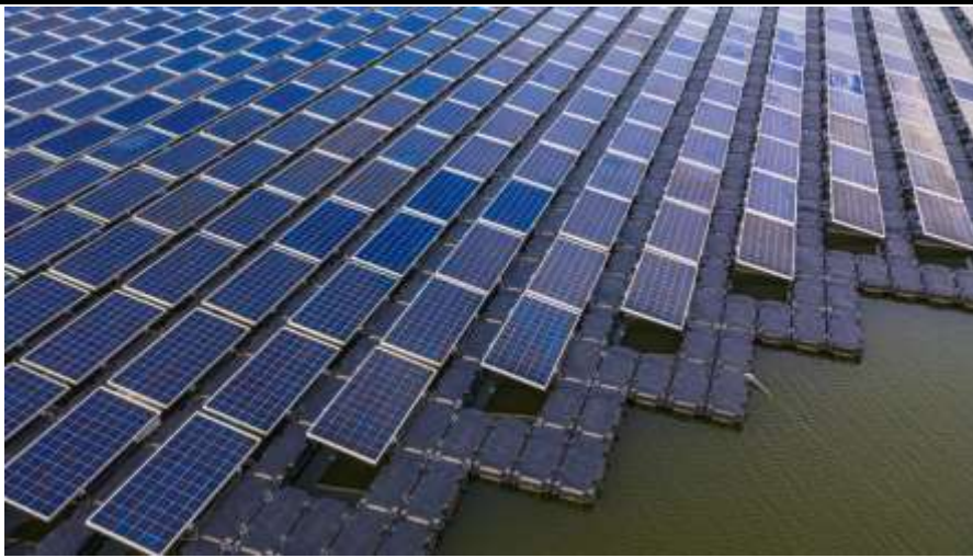
Fig 7. Solar Panels Cohort
