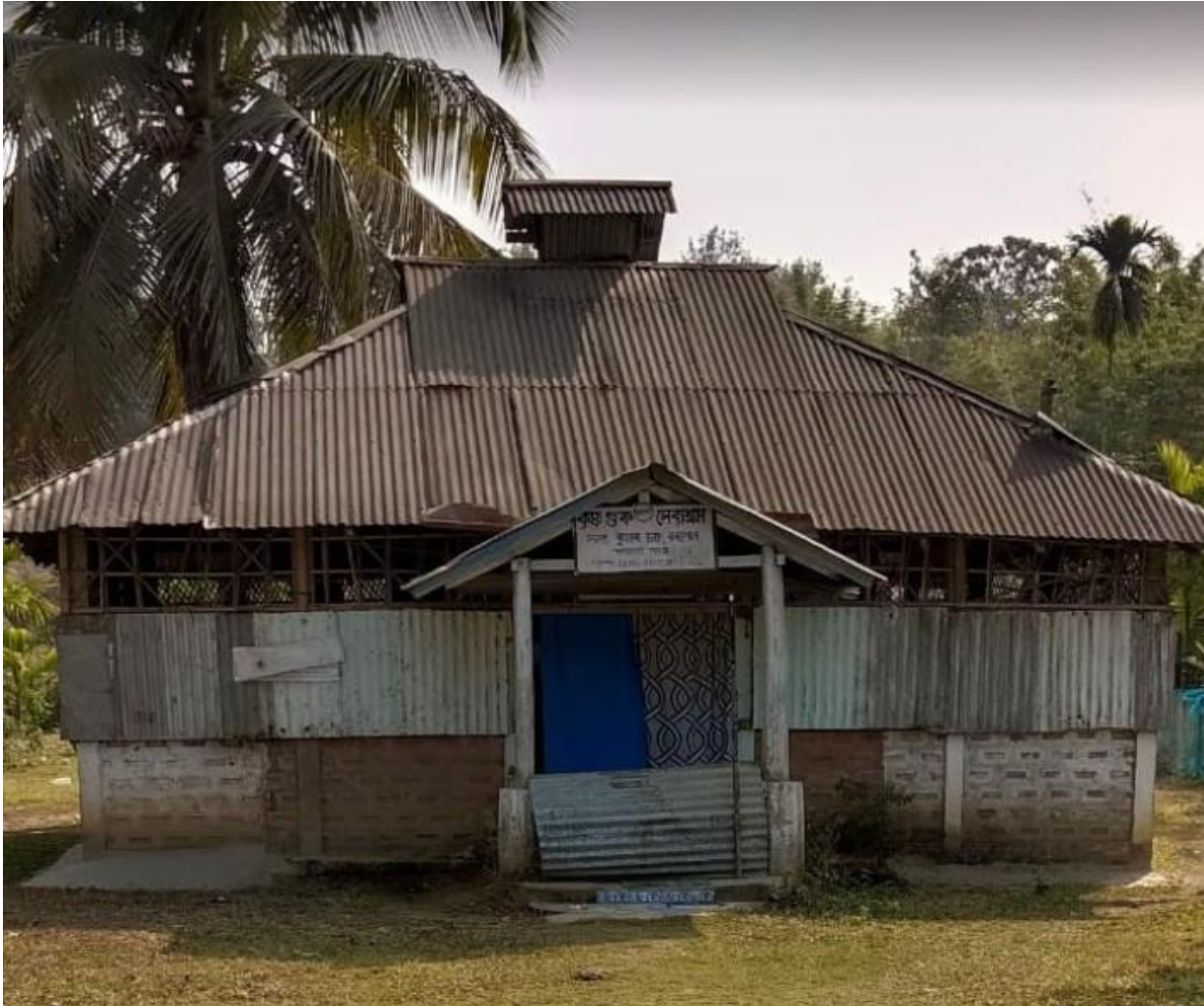
DILAPIDATED STRUCTURE OF ‘‘ KRISHNA GURU SEVASHRAM ‘‘
