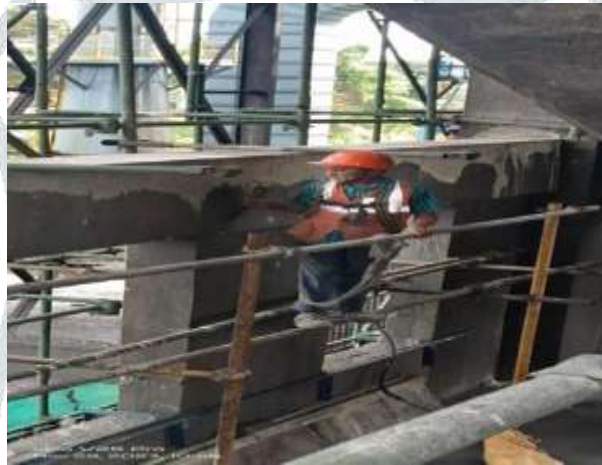
FIG 2(a) UNSTABLE WORKING SURFACE
