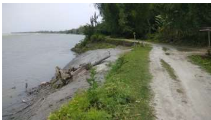
Figure 5 : River embankment erosion of the Brahmaputra
