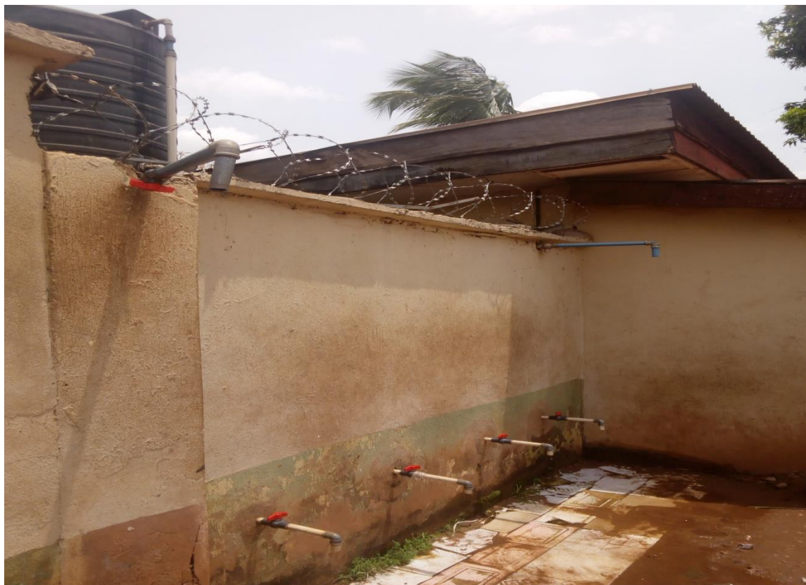
Plate 2: Tap connected from Borehole in Ofiji
