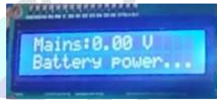
fig-4: Indication of power from battery source
