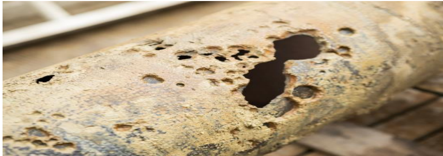
Figure (4): Pitting Corrosion
