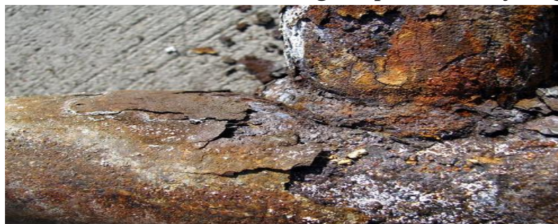
Figure (6): Hydrogen Damage
