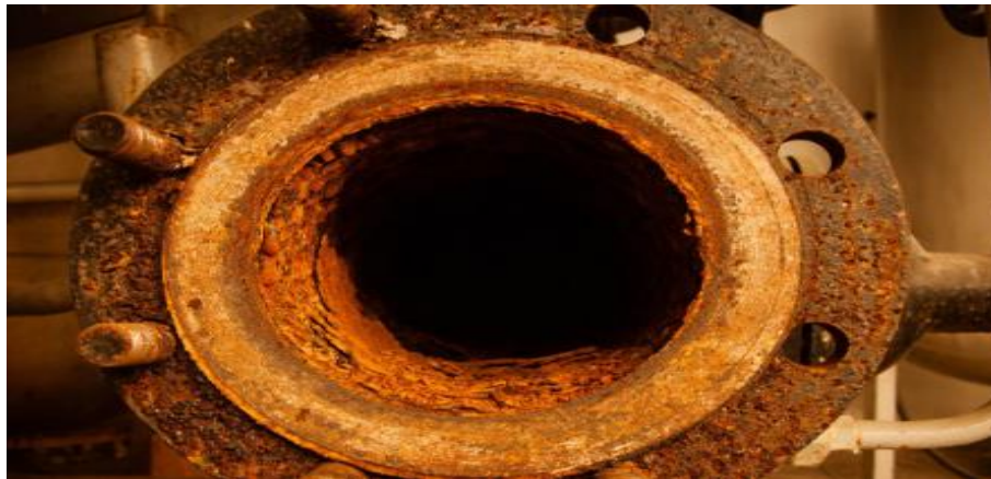
Figure (2): Galvanic Corrosion
