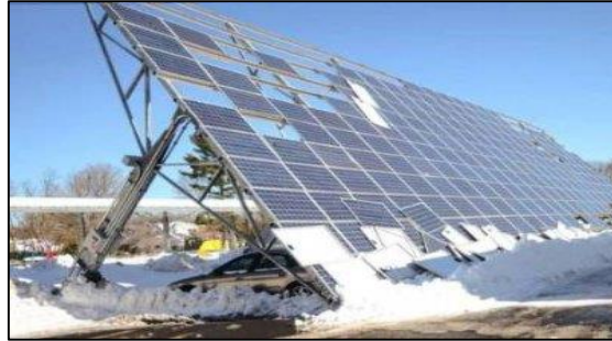
FIGURE8: Panel losses due to wind
