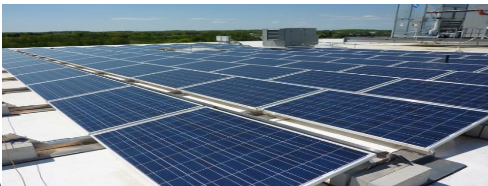
Fig. Solar panel
