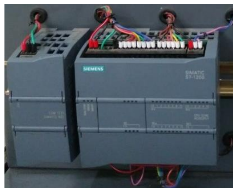
Figure 2 Programmable Logic Control (PLC)
