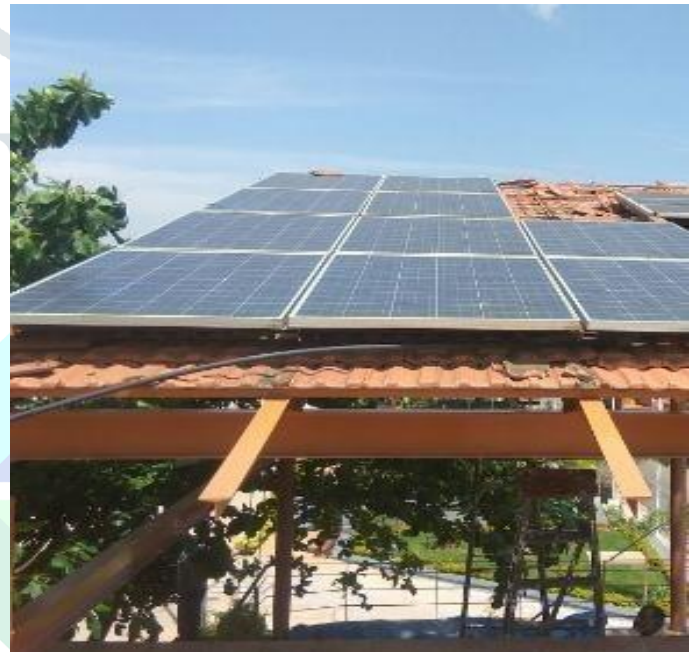
Fig. 3: Solar PV Panels on the roof
