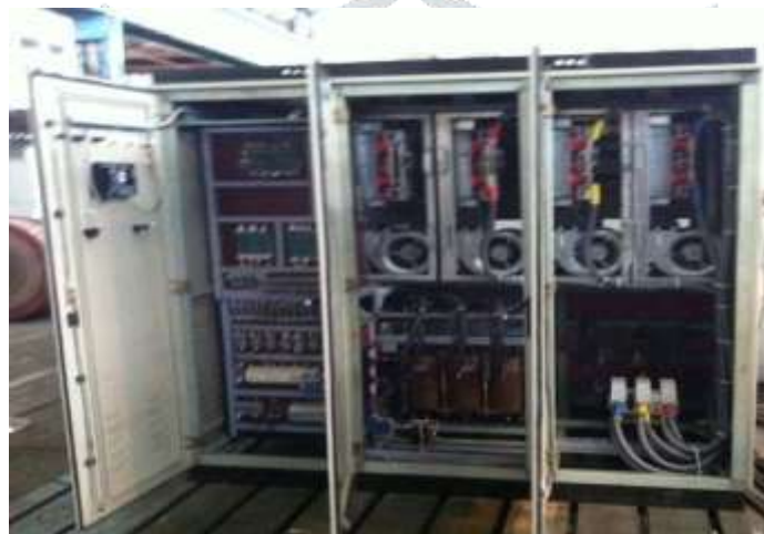
Fig. 3 Inside View of 1MW VFD
