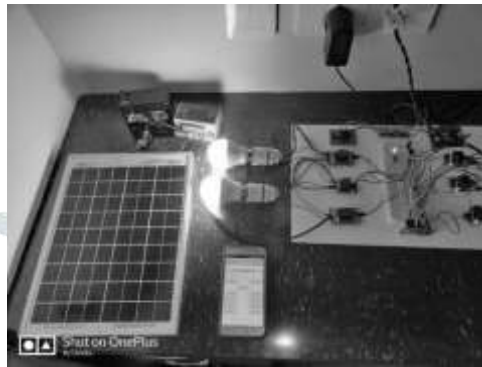
Fig. 3 DC Lights operation using solar energy
