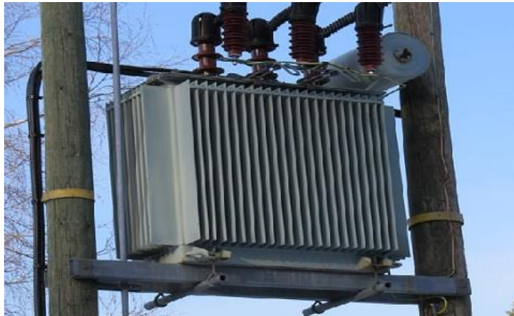
Figure 5: An Actual Image of Distribution Transformer
