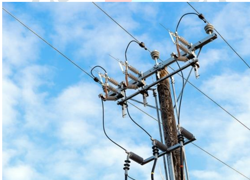
Figure 6: Overhead Transmission line
