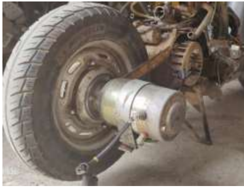
Fig.4 BLDC motor installation
